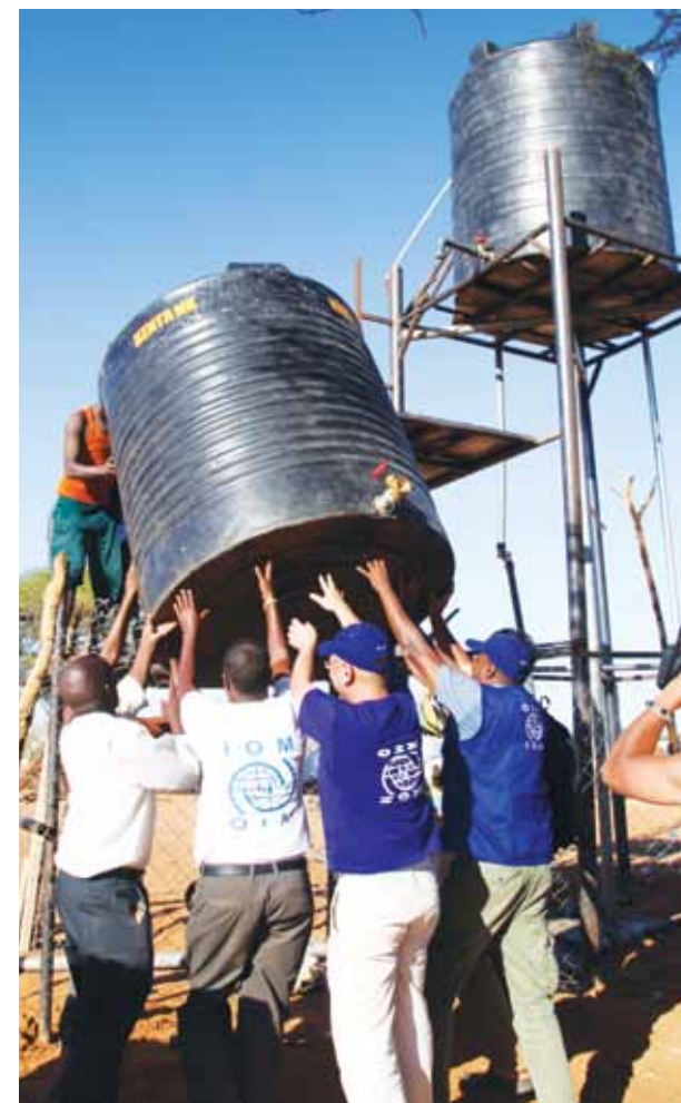
A water tank is set up at Kabasa IDP settlement by the community, IOM and partners. © IOM 2013 (Photo: Kaori Nakasa)
